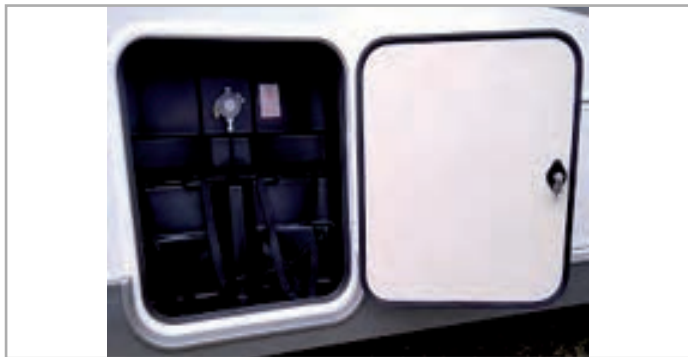
Fig.6.26 - Gas cylinder compartment
